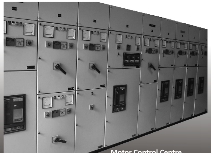
Motor Control Centre
