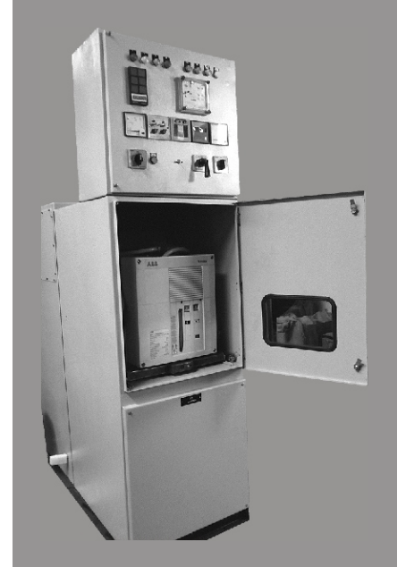
Indoor VCB with ABB Breaker
