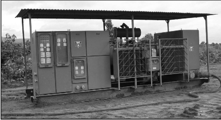
1 MVA Mine Substation
