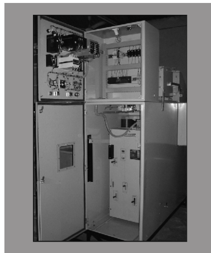
11 KV VCB Panel
