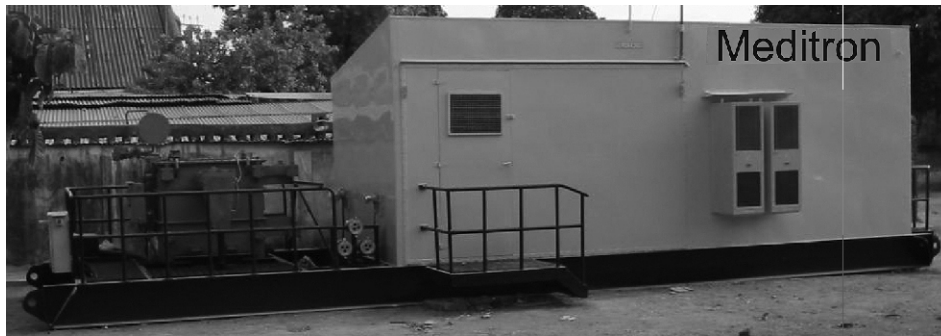
1 MVA remote controlled Substation with SCADA
